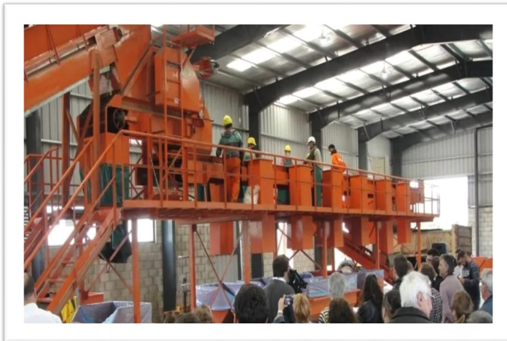
3.2: Waste separation and classification plant.
