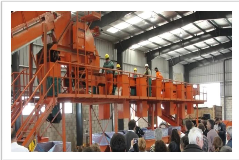
3.2: Waste separation and classification plant.
