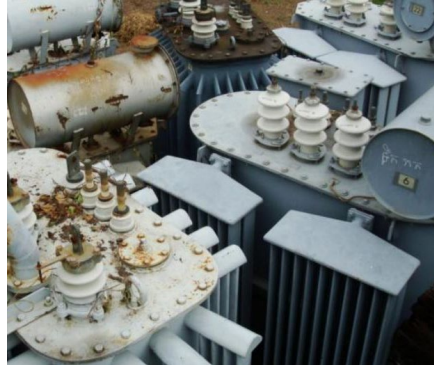
Polychlorinated biphenyl (PCB)-containing transformers classified as metal scrap.
